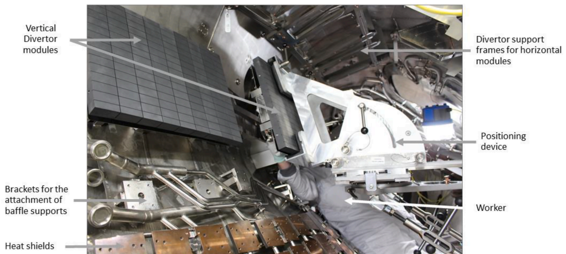
Fig. 3. In this situation, a worker installs a Vertical Divertor module, supported by a position device. Positions for the later assembly of Horizontal Modules, baffles and Heat shields are visible
