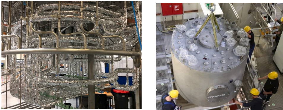
Fig. 7. Piping inside the cryo valve box (CBV) on the left side and view from above during the crane transport of the CVB in the W7-X torus hall
