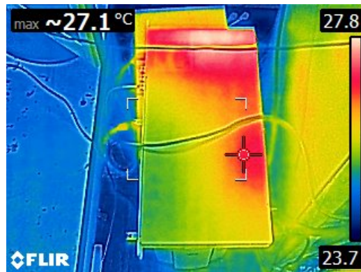
Figure A.10.: Close-Up IR image of the White Rabbit Switch located at the IceCube Lab. This is a different device than the passive patchpanel in the FieldHub.
