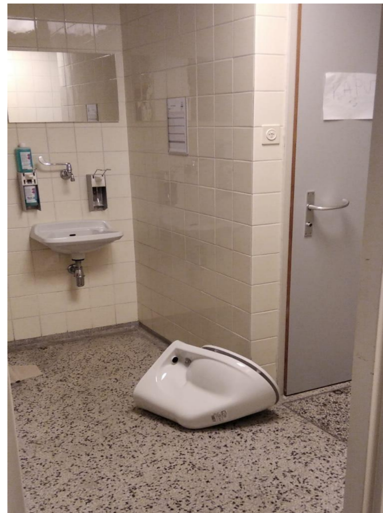
Toilet in a public hospital in Vienna that has been in this state for 6 years. The toilet is in a state of disrepair, with the bowl lying on the floor. This is a clear example of the neglect that some public hospitals in Vienna are facing.
