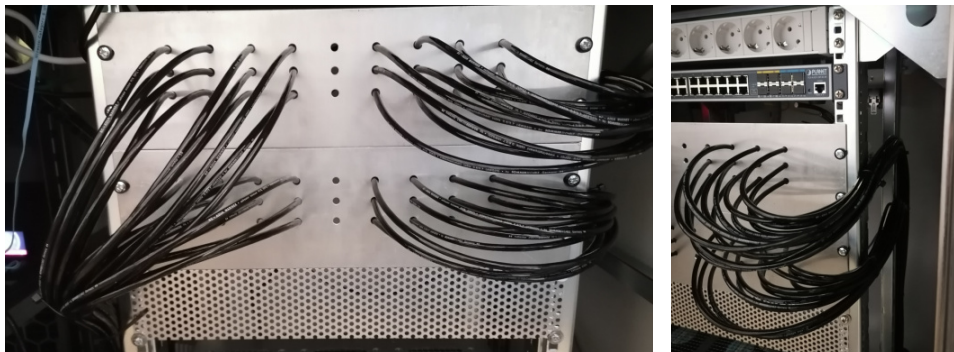
Figure 49 Left: Front view of the cable routing inside a cabinet with 19-inch rack. On the left half the cables are fed from below and on the right half from the back. Right: Photo of the cables fed in a single bundle from the back of the rack to each half of the PhantomHV dummies.
