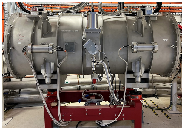
Figure 5: SCU16 installed in the storage ring.
