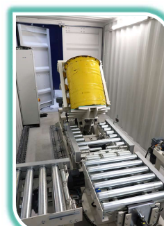
Drum on tipping system
