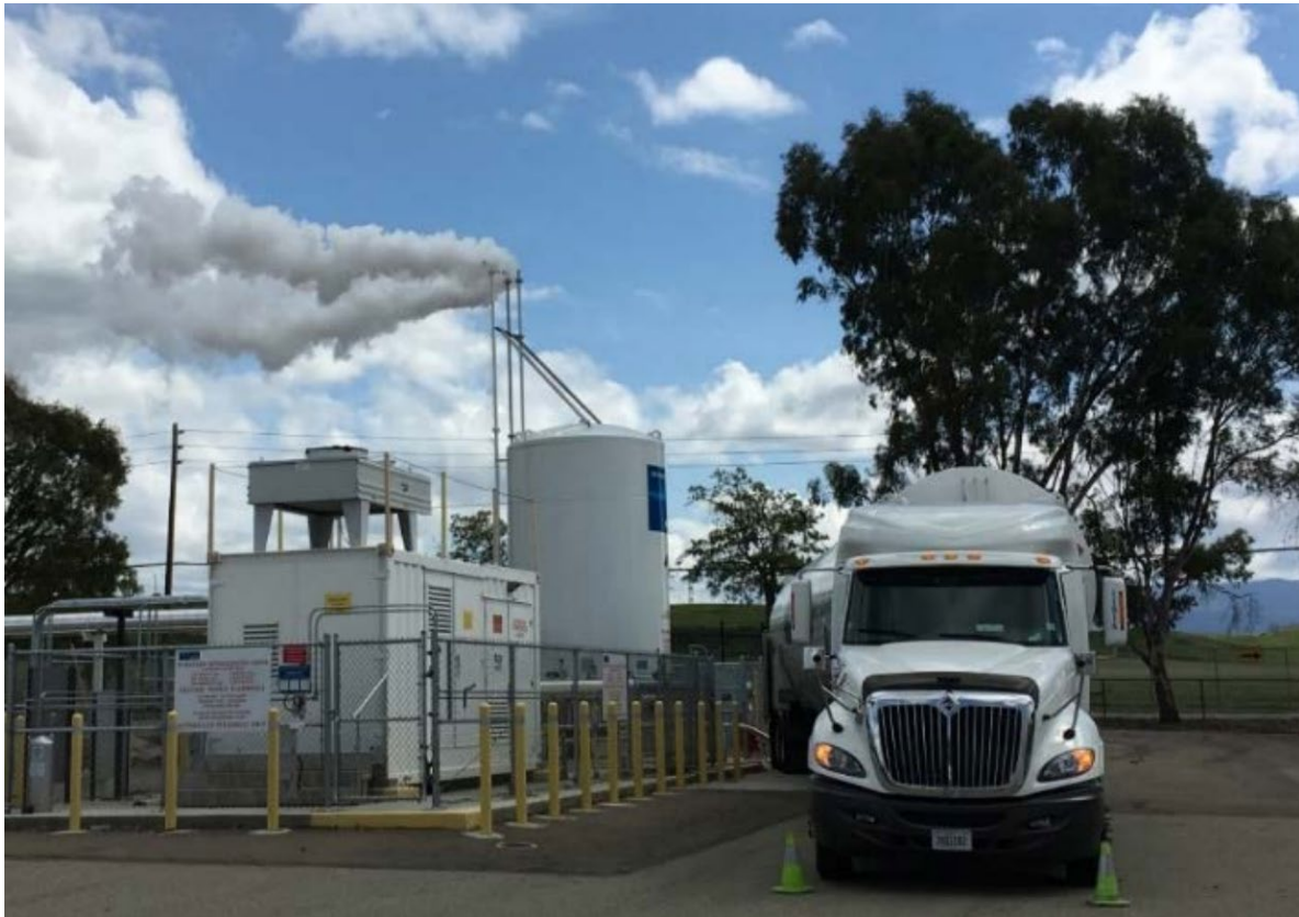
Figure 6.2: Removal of displaced gaseous hydrogen via the chimney of the storage tank during LH 2 delivery. Due to the coldness of the discharged gas, moisture condenses locally from the air and a cloud of fog forms. Source: 13
