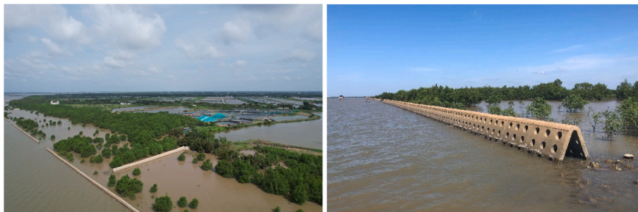
Fig. 1. A section of hollow triangle breakwater TC1 constructed along the coast of Mekong Delta (pictures taken in 2023).
