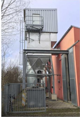
Photograph of the baghouse filter exterior
