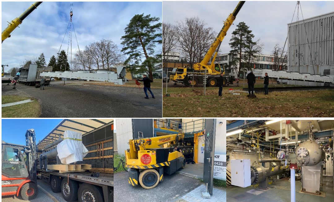
Figure 3: Assembly of the external cooler (top) and the steam generator (bottom) after maintenance before commissioning
