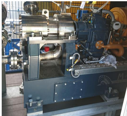
Fig. 4: Turbine with gearbox and generator
