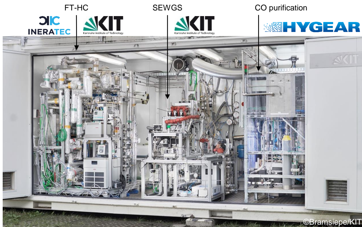
Fig. 5.8: Photograph of the Kerogreen container with FT-HC, SEWGS, and CO purification modules (provided by the project partners INERATEC GmbH, KIT and HyGear B.V., respectively), located at IMVT, KIT, Germany. ©Bramsiepe/KIT
