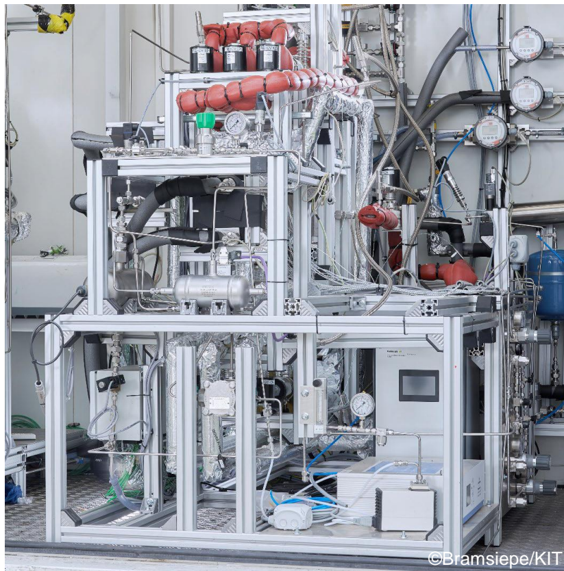
Fig. 5.7: Photograph of the SEWGS module (front view), located at IMVT, KIT, Germany. ©Bramsiepe/KIT
