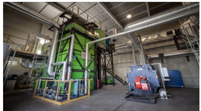
Figure 1: DH boiler room in the town of Lenart, Slovenia Copyright © 2022 Ekoenergo d.o.o.[3]
