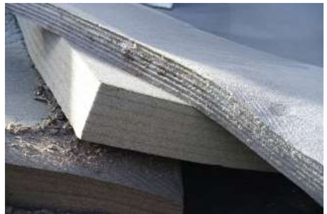
Figure 1: Shrinkage of an insulation material in Marstal - Solites
