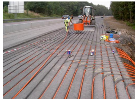
Figure 1. Installed heating pipes in Göteborgsbacken, Sweden, before installation of the binding layer. The figure also shows the connection of the heating pipes to the distribution system (Image source: NCC).
