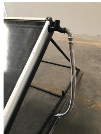
Figure 2: Flexible pipe to adjust slope of the solar collectors
