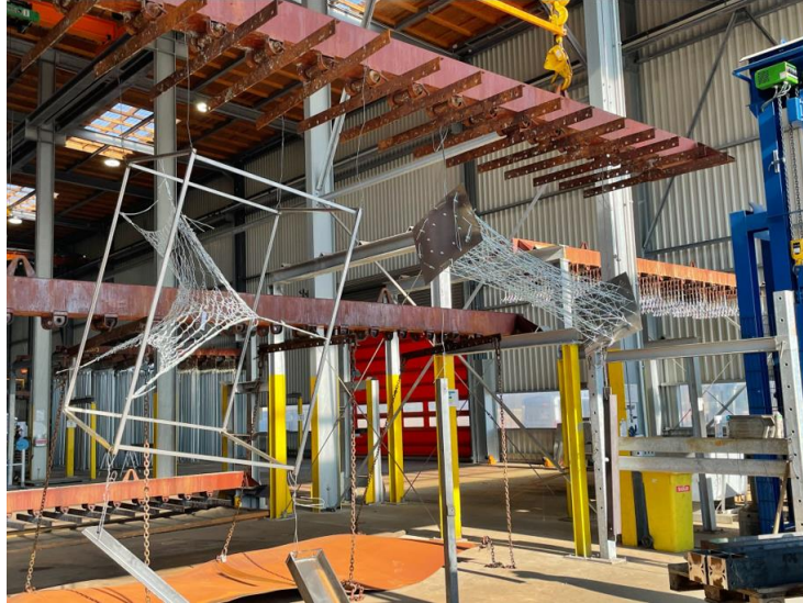
Figure 5. Hot dip bath galvanisation of the final 1:1 prototypes [Photo by Daniel Fischer].
