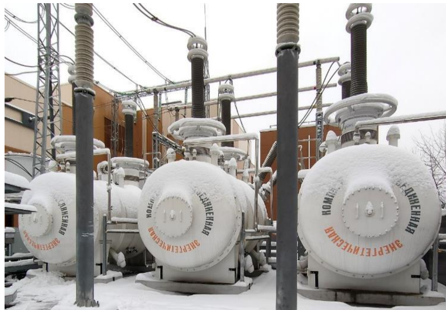
HTS SFCL placement at Mnevniki substation
