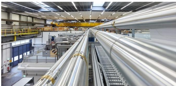
Fig. 2. 87 mm inner-diameter corrugated HE11-mode waveguide transmission lines at ASDEX Upgrade.
