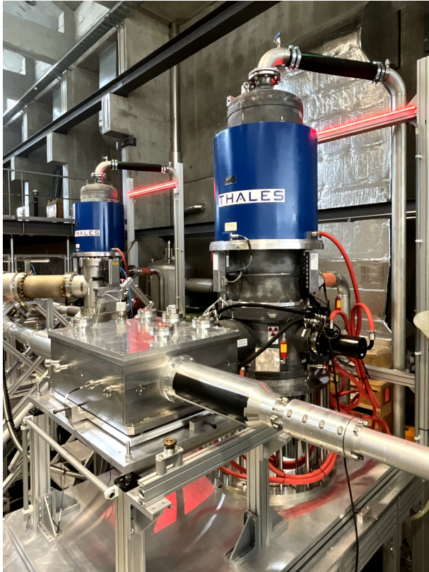
Figure 1. Photo of the two dual-frequency gyrotrons installed in the TCV building. One of the Matching Optics Units is shown in the first plane of the picture.
