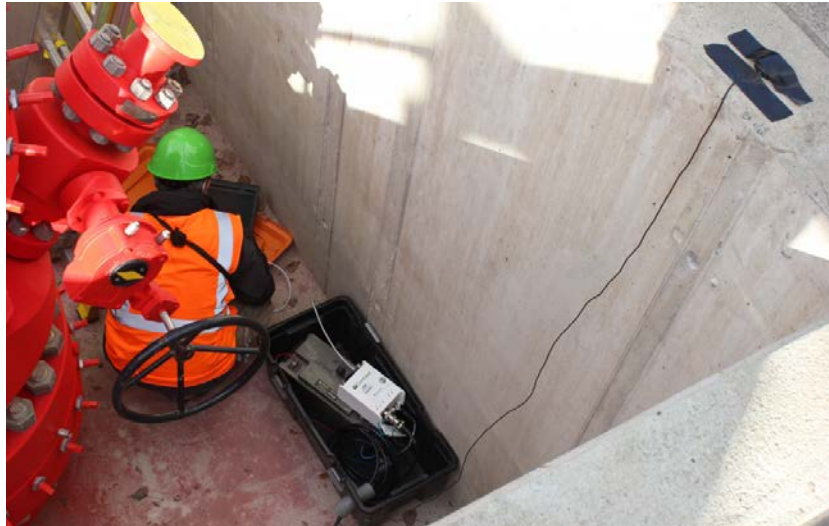
Figure 3-4: Top – Station SLS1. Bottom – Station SLS3, in the cellar of the well SLS-Th2a.
