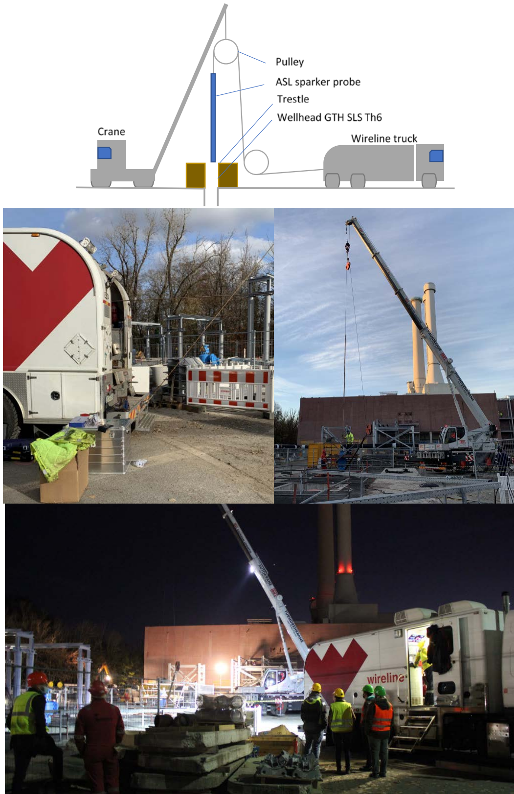
Figure 3-2: Schematic (top) and pictures (bottom) showing the deployment and the routing of the AST assembly in the Th6 borehole.
