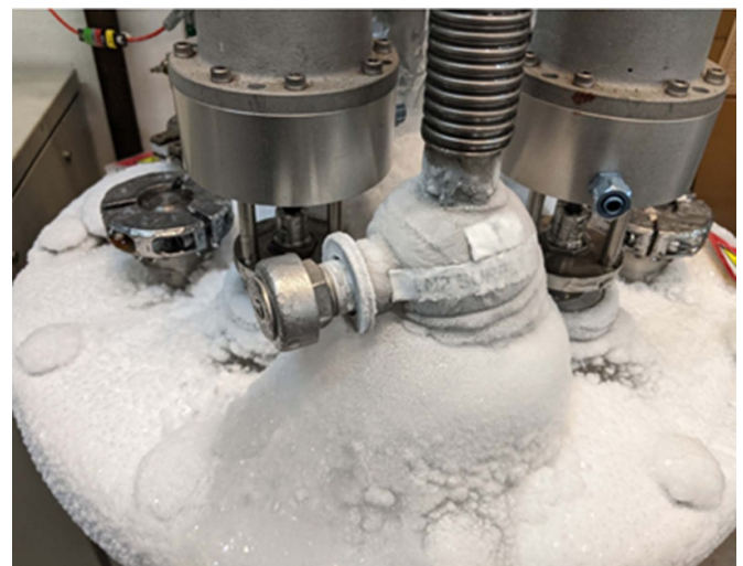
Figure 21. Build-up of ice around cryogenic plant. Such condensate and ice requires careful management due to the potential for preferential exchange of hydrogen for tritium into the water or ice.
