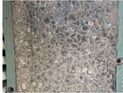
Washed concrete track
