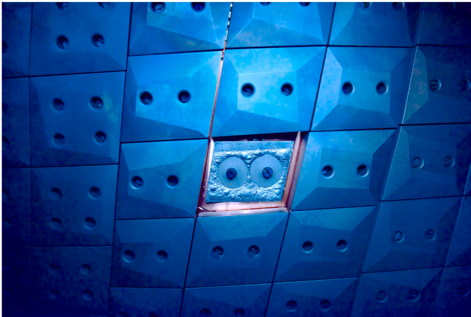
Fig. 2. The beam dump area around the damaged tile.
