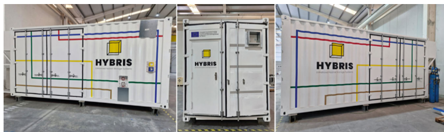
Fig. 7 Hybris containerized hybrid battery energy storage
