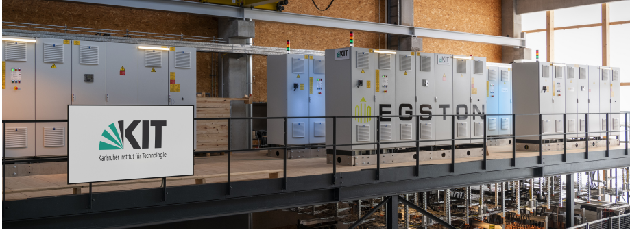
Figure 3.3: Five 200 kVA GAMP6 Egston switched-mode power amplifiers (1 MVA in total).
