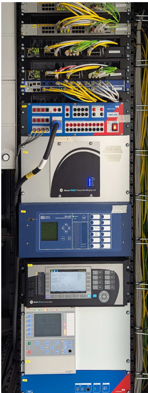
Fig. 3: View of the KASTEL Security Lab Energy testbed racks housing (from top to bottom) network switches, multivendor IEDs, Merging Units (MUs), Intrusion Detection System (IDS).
