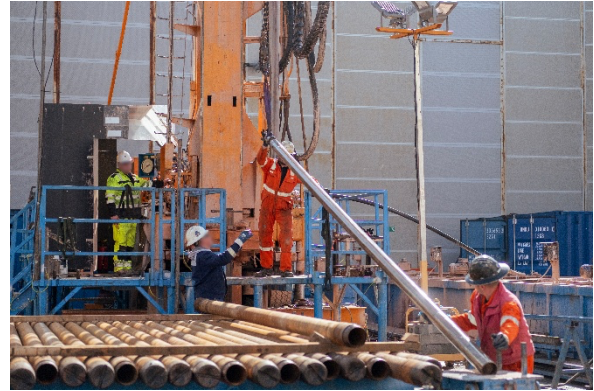
Fig. 8: Drilling of GLB-1. The borehole reached a depth of more than 500 m and was fully cored. The drilling results form the basis for the site evaluation and assessment of whether the Tromm location is suitable for the planned underground research lab GeoLaB.
