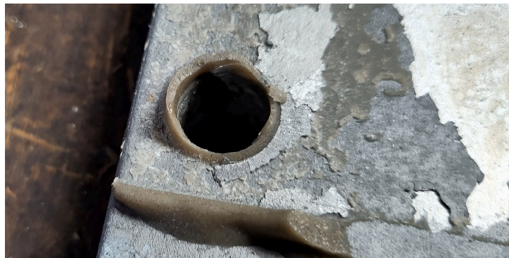
(c) Detail view: bolt hole with local tear-off of the zinc coating.
