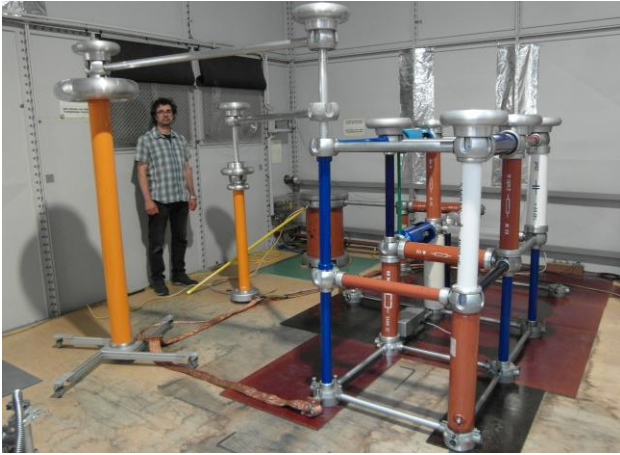
Figure 5 High voltage test setup.
