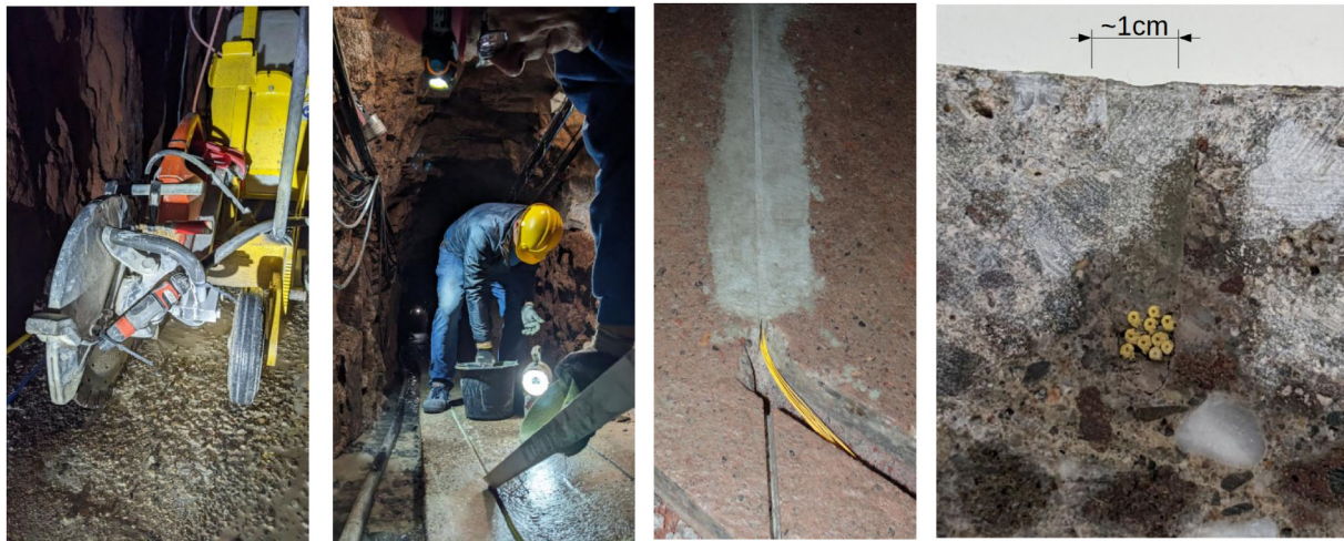
Figure 2. A 10 mm wide and 10–20 mm deep groove has been cut into the concrete floor of the front part of the gallery (see Fig. 1). Eight single-fiber patch cables, each of them being 0.9 mm thick (see Fig. 3), run in parallel in the groove. The groove has been filled with non-shrinking cement. The rightmost picture shows a cross-section of a preliminary test installation of 10 cables.
