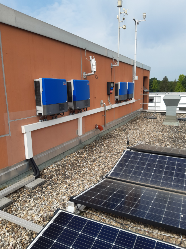
Figure 3.4: Picture of the four inverters of the rooftop PV system located outside on the northern wall of the roof-exit hood.
