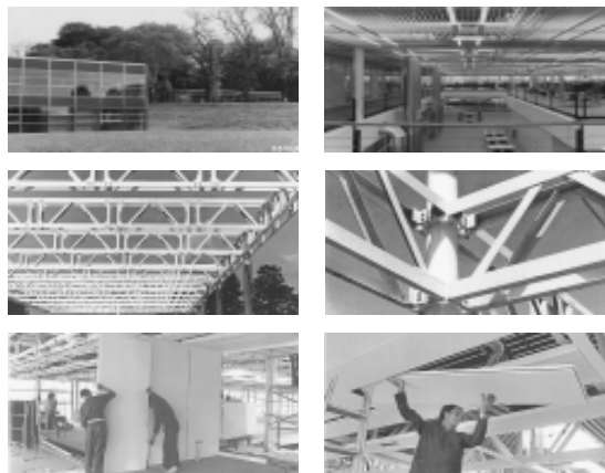
Figure 1: The Swiss railroad's instruction building in Murten, CH in the MIDI construction system. Exterior and interior views, MIDI construction, detail of support column, assembly of interior wall system and suspended ceilings. All construction components used can be dismantled, and their configuration can easily be changed. The building was completed in 1982 and has been renovated four times since.
