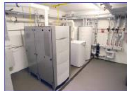
A Vaillant fuel cell heating appliance, Oldenburg, Germany.
