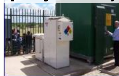
A PlugPower GasCore Fuel System in South Africa provides back-up power for telecommunications.
