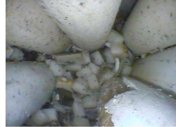
blockage at elevation 910 mm
