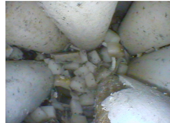
blockage at elevation 910 mm
