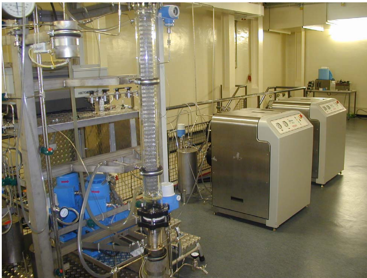
Fig. 2: View of the Experimental Facility for Water Detritiation at TLK
