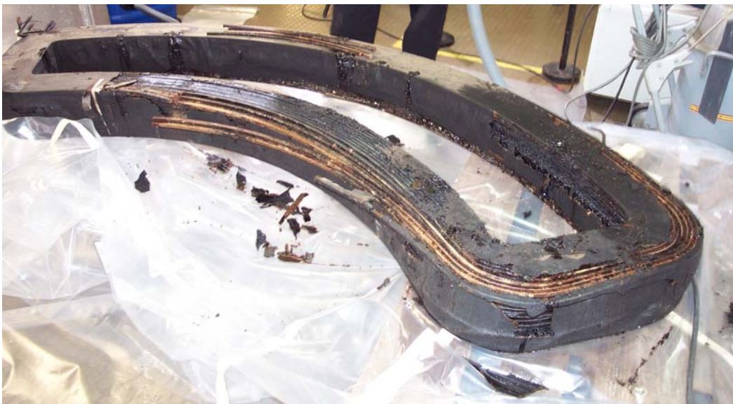
Fig. 3: Damaged lower induction coil.
