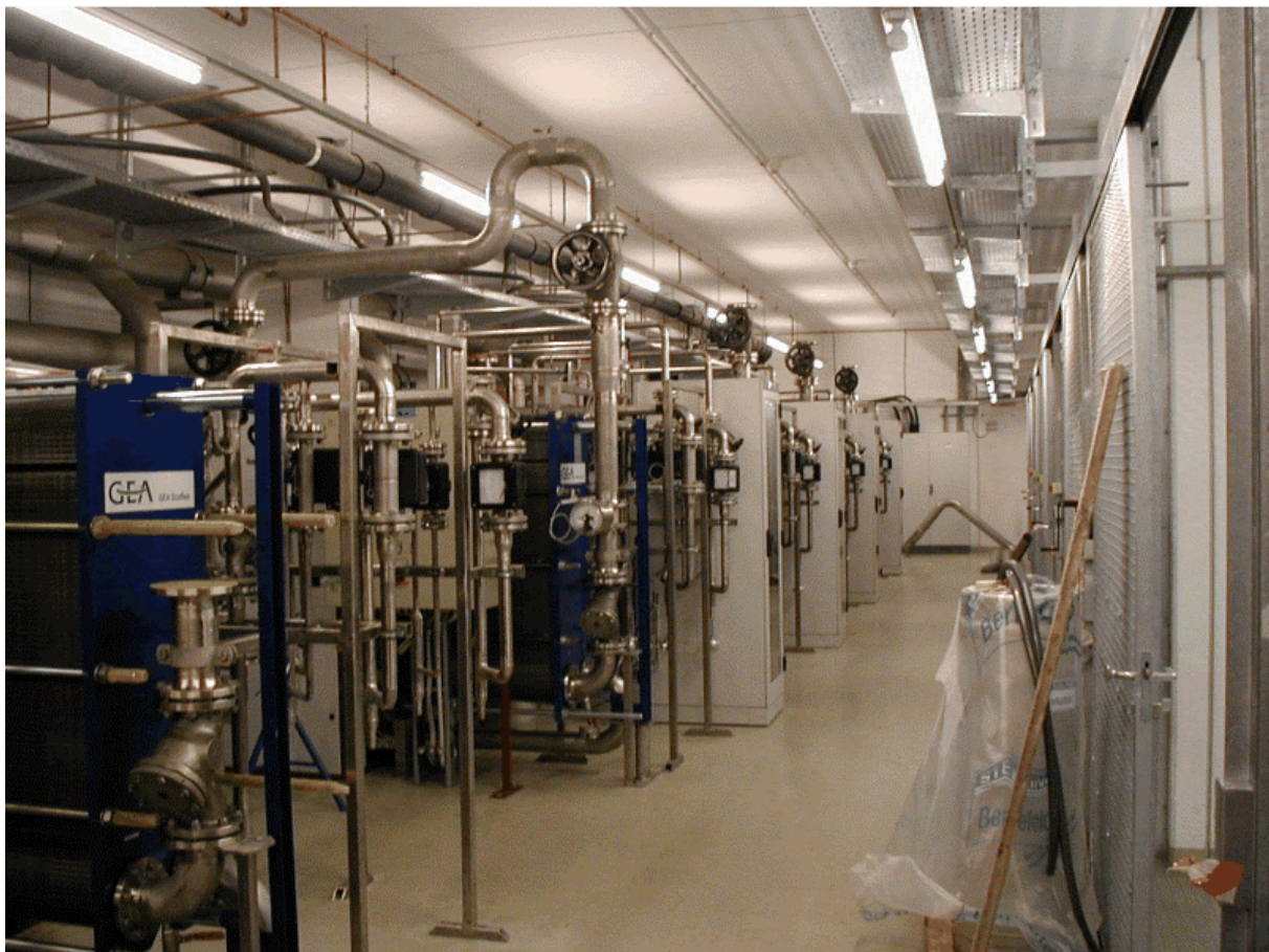
Fig. 5: Gyrotron water cooling modules.
