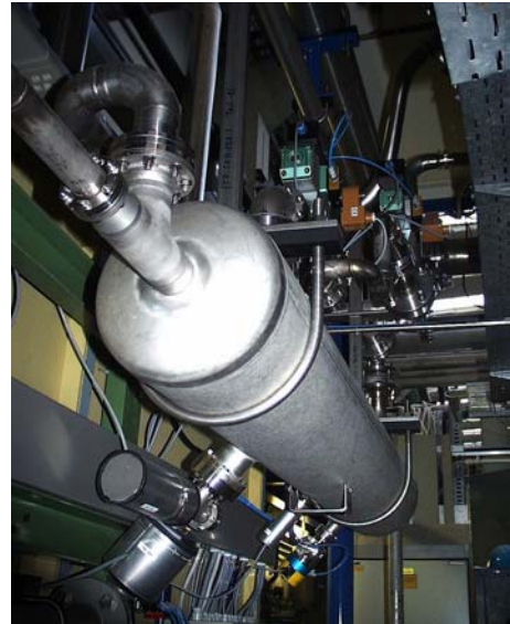
Fig. 2: New buffer tank in the exhaust line.
