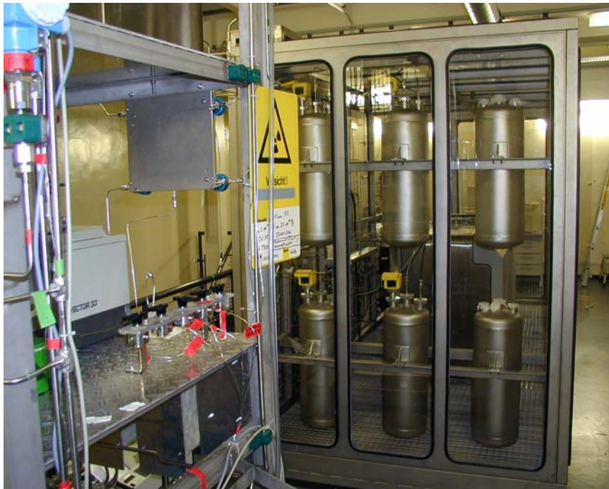
Fig. 2: Ventilated enclosure for the electrolysis unit and feeding vessels.
