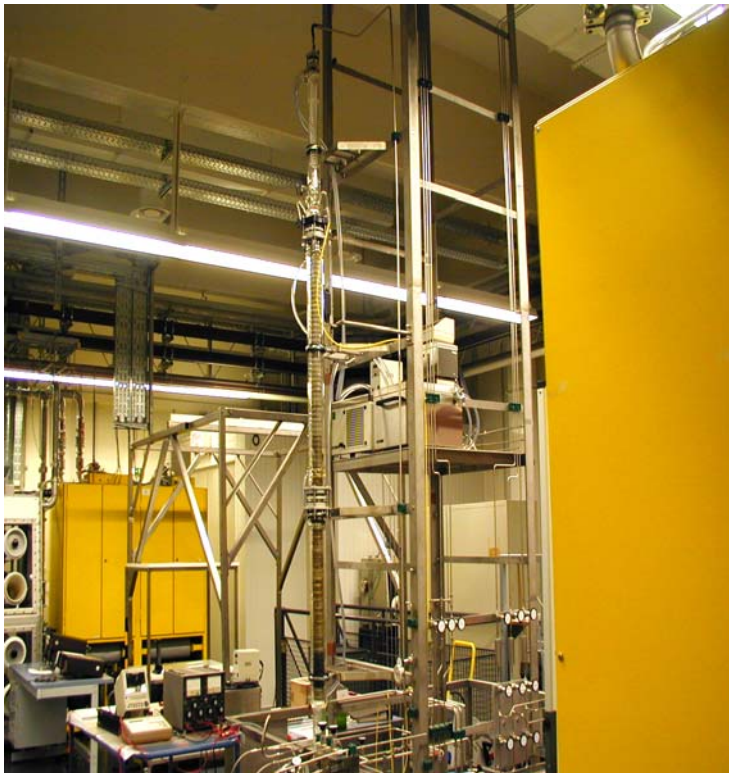
Fig. 2: Oxygen stripping column at TLK.
