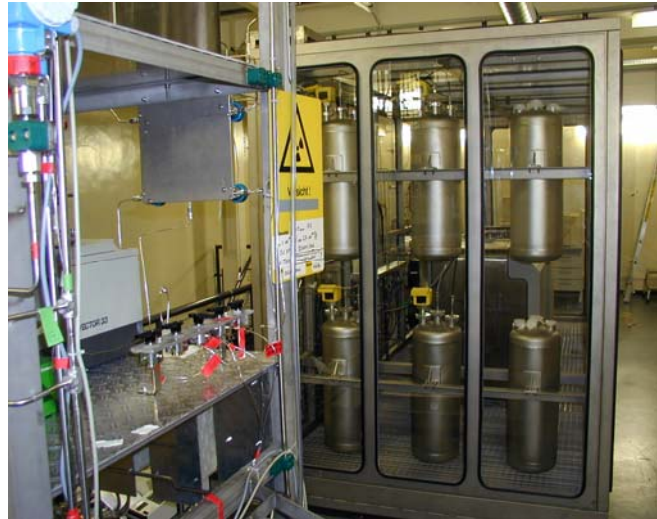
Fig. 3: Ventilated enclosure for the electrolysis unit and feeding vessels.
