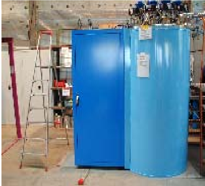
Fig. 3: The refrigeration unit for TRENTA facility.
