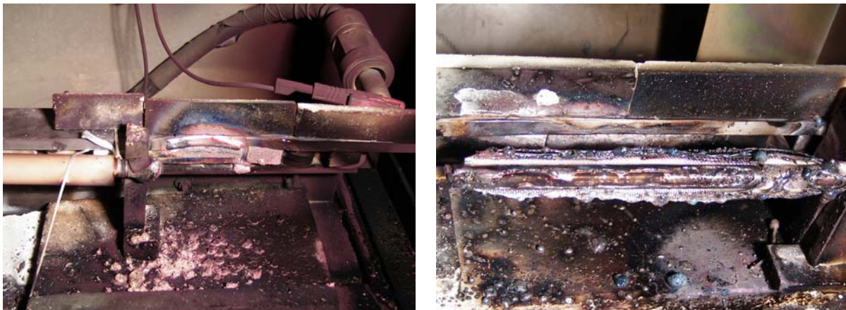
Fig. 5: Photographs taken after arc experiments. The left picture was taken after the backward experiment VA1005 (560A, 22kW). The conductor was completely molten and there is considerable damage to the ground rail. The right picture was taken after the forward experiment VA1010 (750A, 30kW). The conductor insulation and steel jacket are cut, however the copper core is mostly undamaged. The ground rail shows only slight burning traces although the arc power was about 50% higher than in VA1005. This means with regard to safety questions, the backward mode is obviously the more dangerous one.
