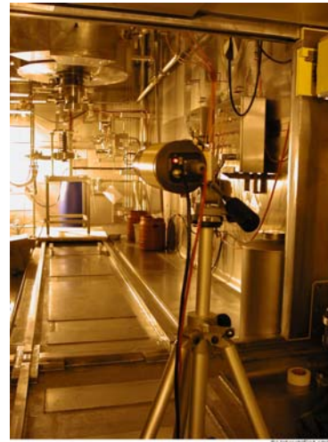
Fig. 4 Thermovision camera in the hot cell V3 viewing into melter cell V2
