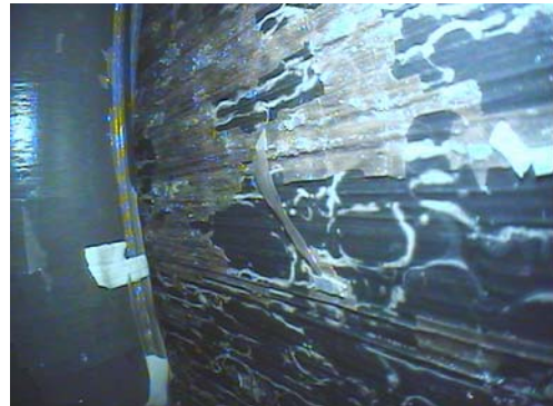
spallations at shroud at 400 mm
