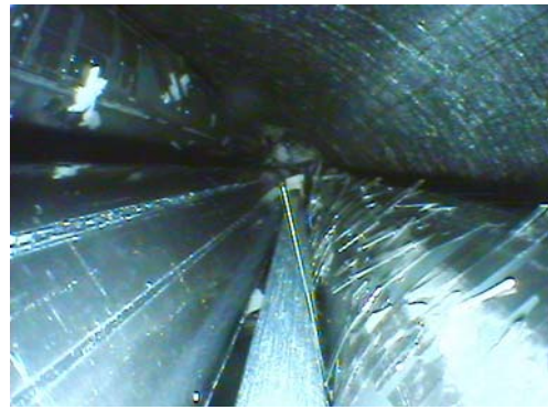
spallations at rod 27 at 450 mm
