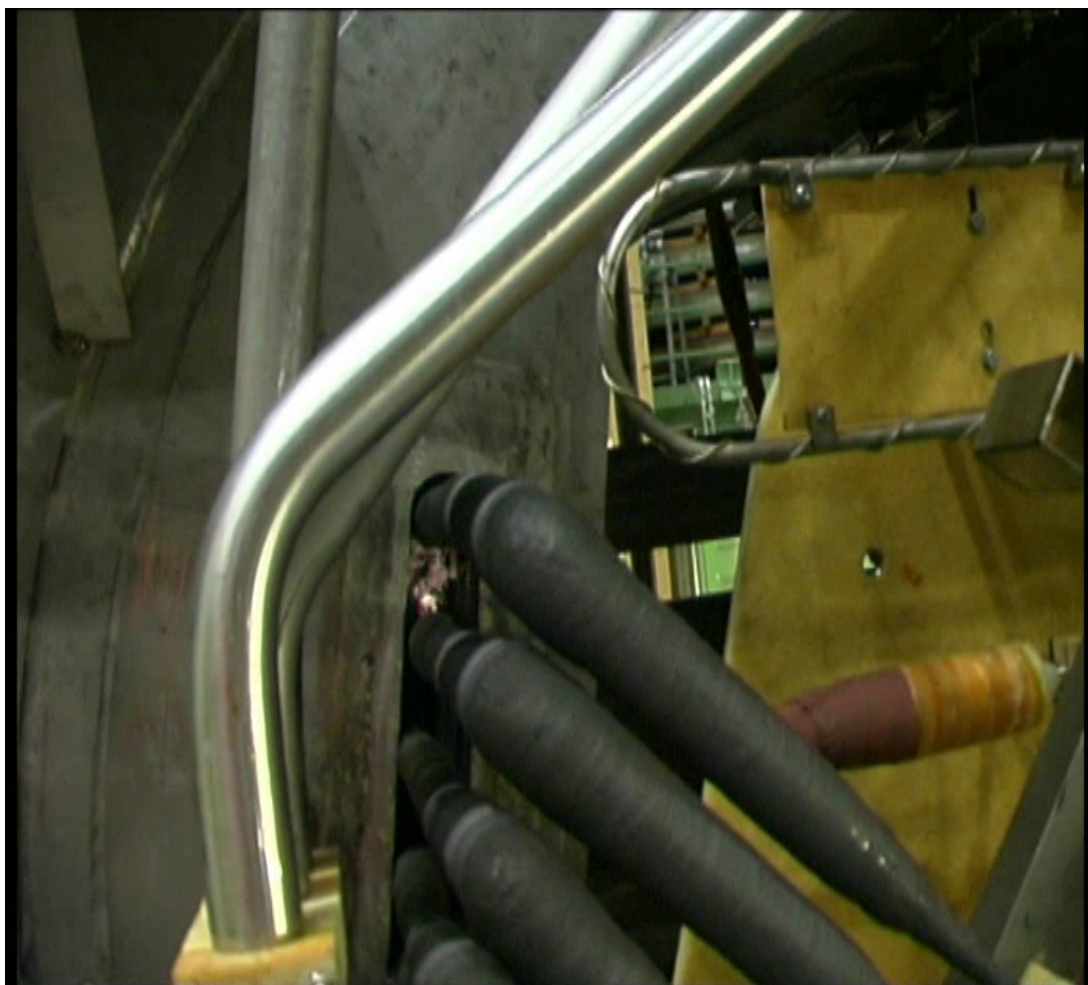
Fig. 6-15 Flash above the second tube counted from top at the inner upper slot of the helium inlet tubes.
