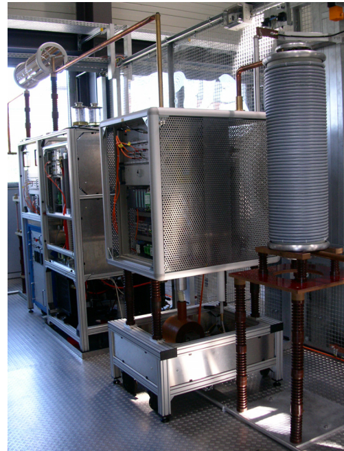
Fig. 5: Complete modulator/crowbar system installed in the gyrotron hall in Greifswald.
