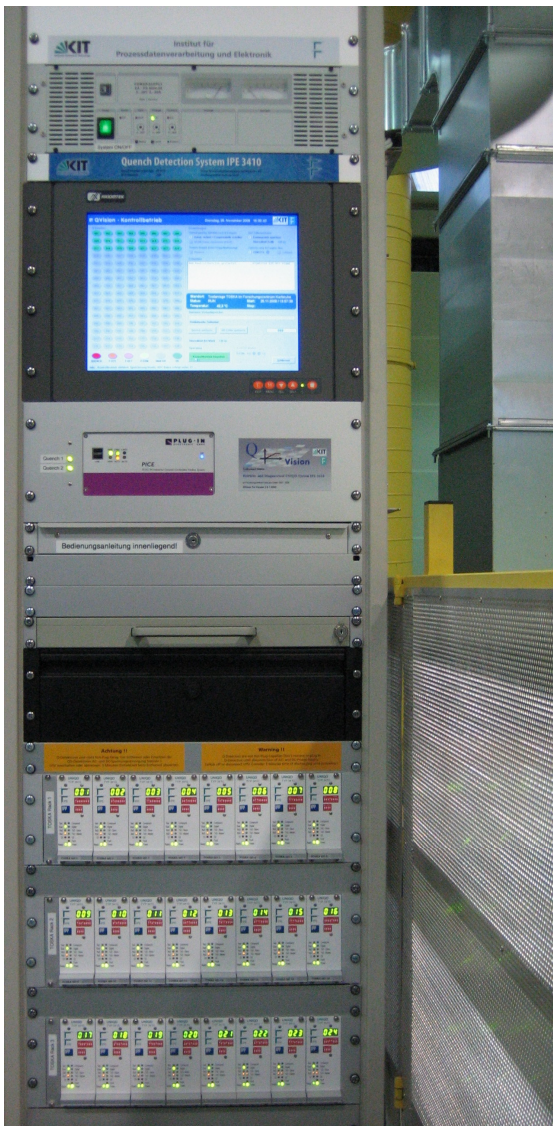
Fig. 6: Quench Detection system at TOSKA consisting of:
