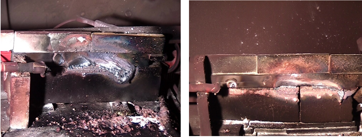
Fig. 4: Damage after RB0303 (left) and RB0508 (right): Although the total power during RB0508 was more than twice the total power during RB0303 (while the burning time was only 30% shorter), the damage to the ground rail is somewhat weaker. The jet-like arc column distributes the power away from the ground rail and expands the structure side spot there which reduces structure damage. One objective of the experiments was to find out about such special behavior of busbar arcs and its relevance for safety questions.
