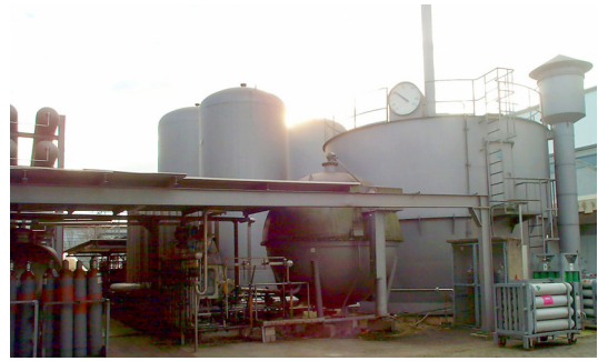
Fig. 3: Helium storage system.
