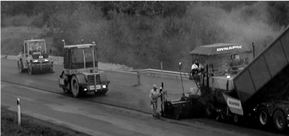
Fig. 4-16. Fleet of a paver and two rollers equipped with ribbon-based systems during OSYRIS worksite tests.
